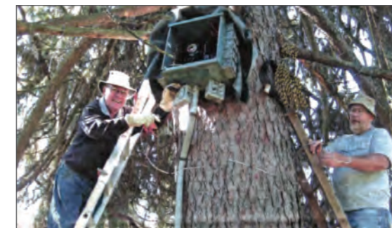
Russell McQuate and Charlie Holt inspect the electrical service on the Community Christmas Tree located at the Wooster Cemetery.
